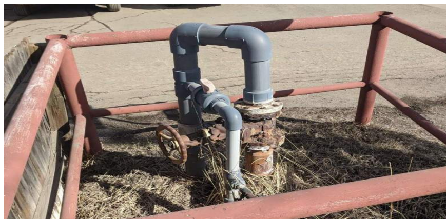
Figure 3. Corroded Well Head
